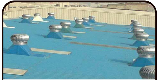
Air Operated Ventilators
